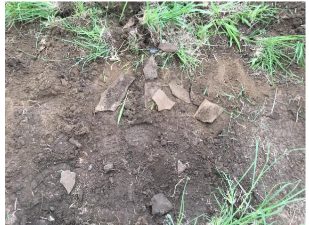
Photo 10. Asbestos containing fibre cement sheeting
