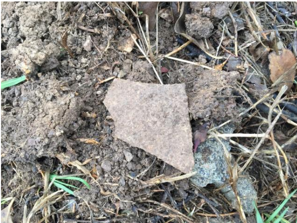
Photo 9. Asbestos containing fibre cement sheeting
