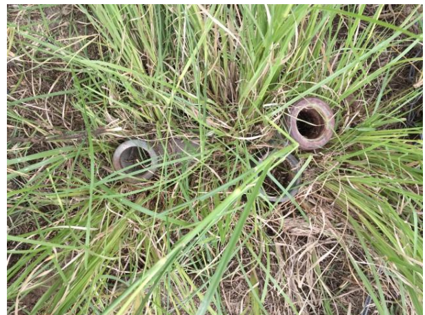
Photo 6. UST fill points near the base of the vent pipe
